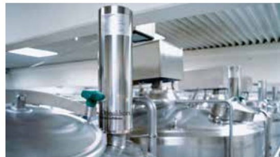
Filter housings for the aeration on storage tanks
